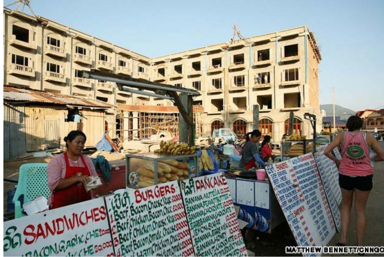
A woman sells pancakes in front of the construction of a huge hotel complex. With such a massive increase in visitors, guesthouses and hotels are being built at a rate of one a week.
